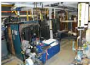
Mackenzie Hospital boiler room
