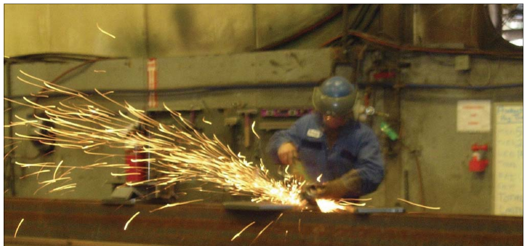
Steel for the Fort St. John Hospital and Residential Care Project being fabricated at Whitemud Ironworks in Edmonton, Alberta.
