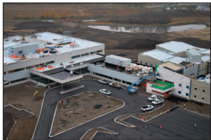
An aerial shot showing the progress of the Fort St. John Hospital and Residential Care Project before the first snowfall of 2011. Photo: Tom Sparrow
